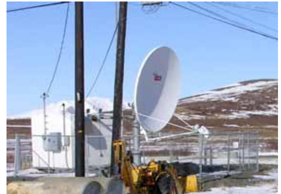
Typical Telecommunication Earth Station in Southwest Alaska
